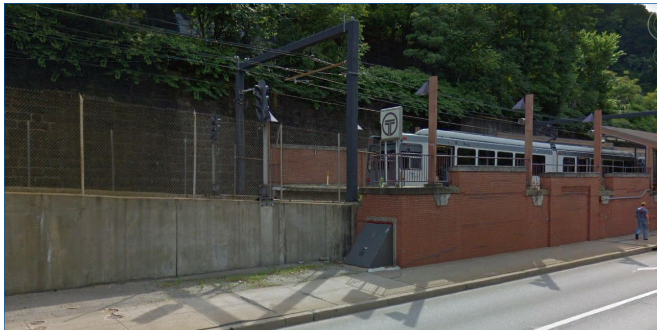
A view of the existing east end of Station Square transit center. There is a bulkhead that accesses electrical infrastructure as well as minimally effective station branding.
