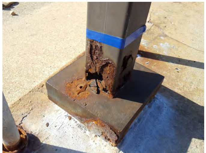
Examples of corroded metals at existing stations. Top: Steel and aluminium combined in a windscreen assembly with paint failing where steel meets the platform surface. Bottom: A factory painted light post with significant corrosion from salt exposure.
