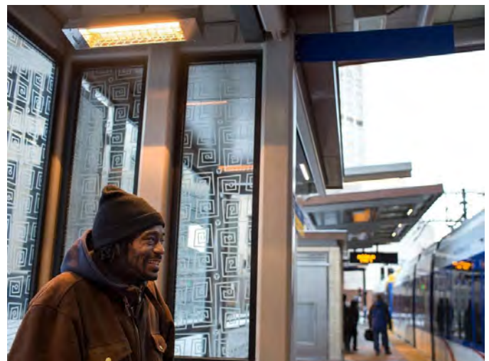
New canopy heaters at Central Station, St. Paul
