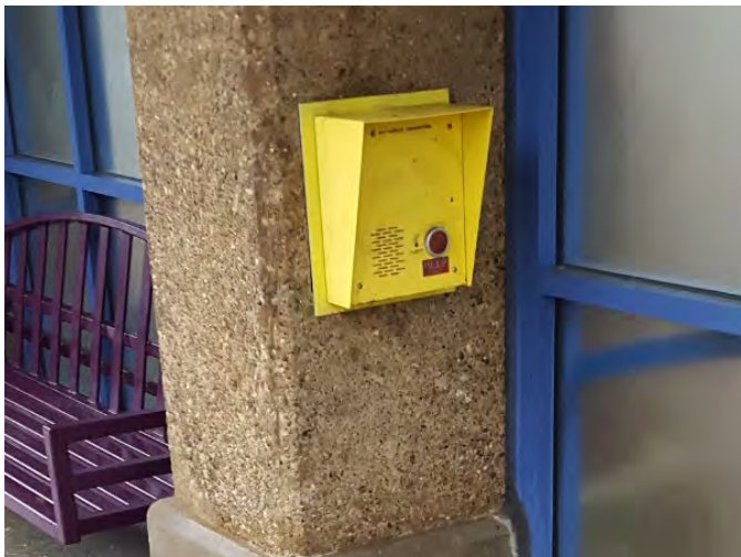
Existing ECB integrated into the structural column of the canopy structure along the Blue Line, Pittsburgh.
