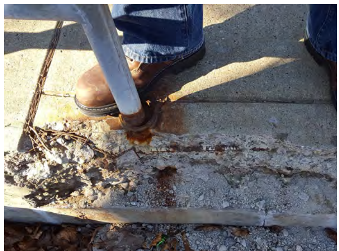
Example of Corroded Concrete at an Existing Station.
