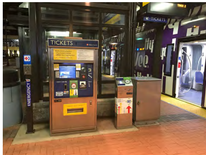
On-platform, covered ticket vending machines, placed with validator and emergency button, at Government Plaza Station, Minneapolis.
